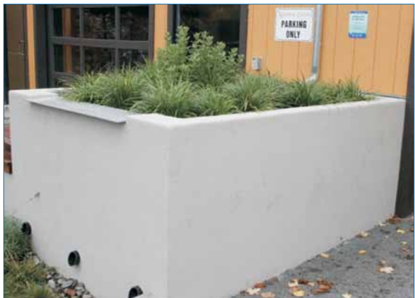
Figure 4 A disconnection planter serving a commercial property (note outreach plaque on the wall) (courtesy DS 7 Photography)
